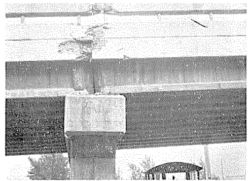
Fig. 17 Spalling of concrete at deck level
