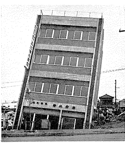
Fig. 2 Reinforced concrete building tilted over and subsided
