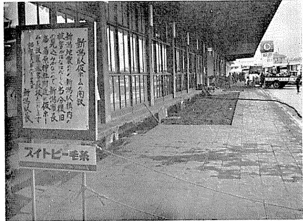
Fig. 27 Subsidence of foundation material
