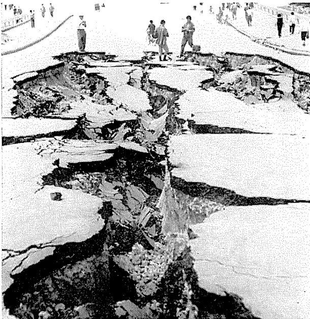
Fig. 5 Extensive subsidence of embankment of Shin-Showa Bridge
