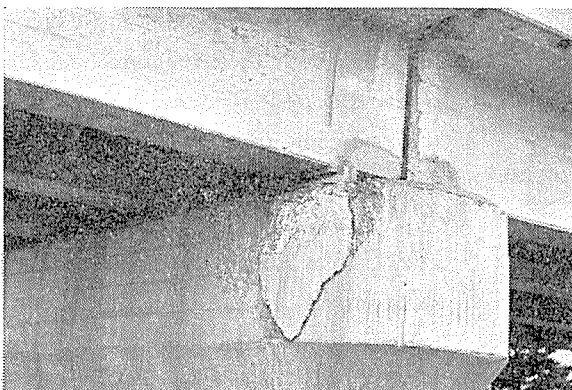
Fig. 16 Cracks on the bearing surface and front surface of the pier : too narrow bearing area and not reinforced enough
