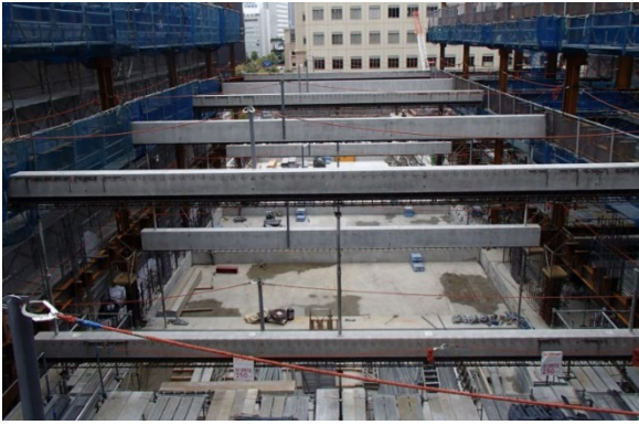
1) Half of the girders were installed at the same time as the steel erection
